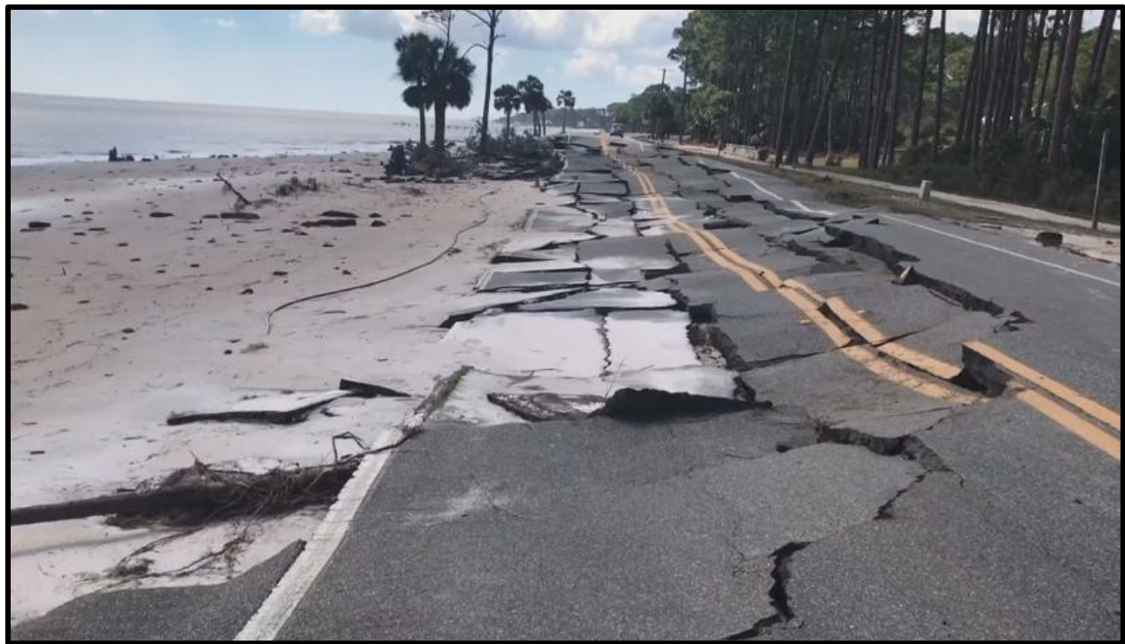
Storm surge damage to highway 98
